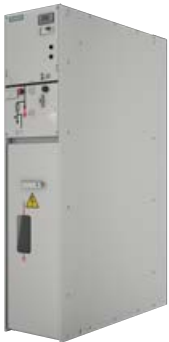
Transformer panel, type T
