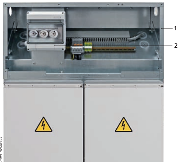
Low-voltage niche of a billing metering panel type M, open cover
